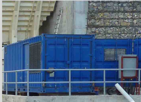
Power is by hydraulic pumps driven by either an electric motor or a diesel engine. Controls are handled by a PLC making adjustments simple. With continuous monitoring of all key items.
